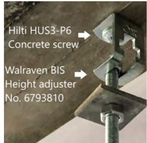
C-clip detail used previously by JEG electrical on satellite hospitals and NRH
