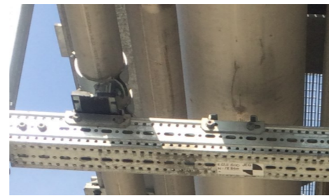
Pipe shoe and guide assembly bolted in place
